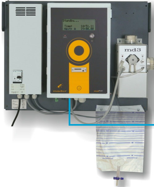
ANALYSER WITH GAS CONDITIONING UNIT #1
